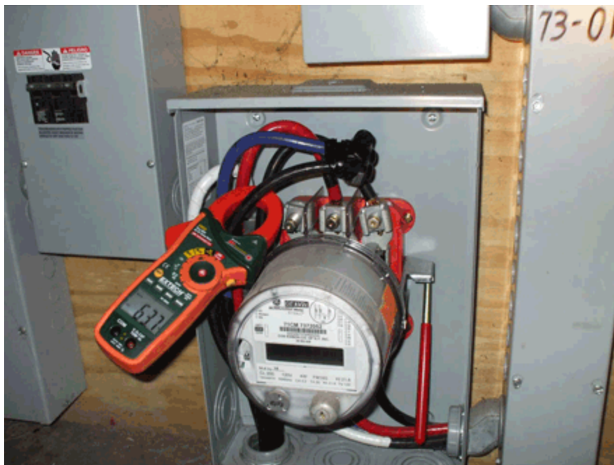
An example of a meter in which the phase with the most load was rerouted around the meter.
